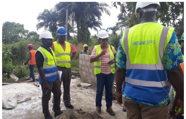
UNOPS and stakeholders jointly conducting routine project site inspections. Photo: ©UNOPS Liberia
